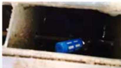
'Nose' in the feeder entrance (viewed from underneath)
